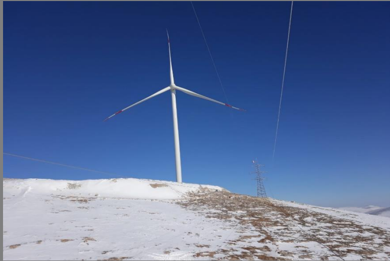
*154 kV SINGLE CIRCUIT 1272 MCM ARDIÇLI RES- BAĞLAR RES ENERGY TRANSMISSION LINE Konya /TURKEY
