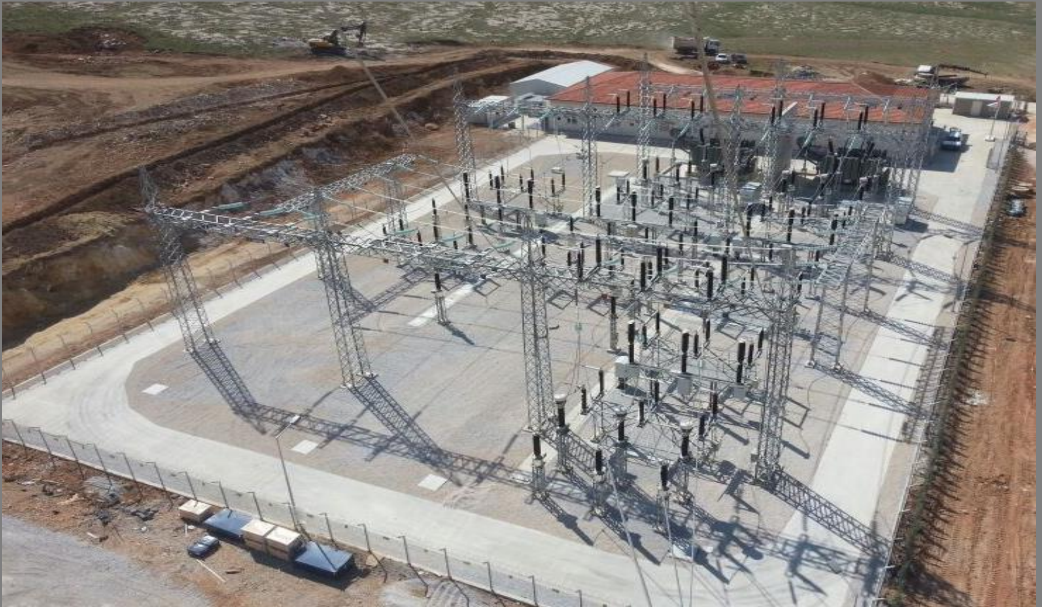
154 KV ARDIÇLI RES SUBSTATION CONSTRUCTION ELECTRICITY INSTALLATION, TESTING AND COMMISSIONING
